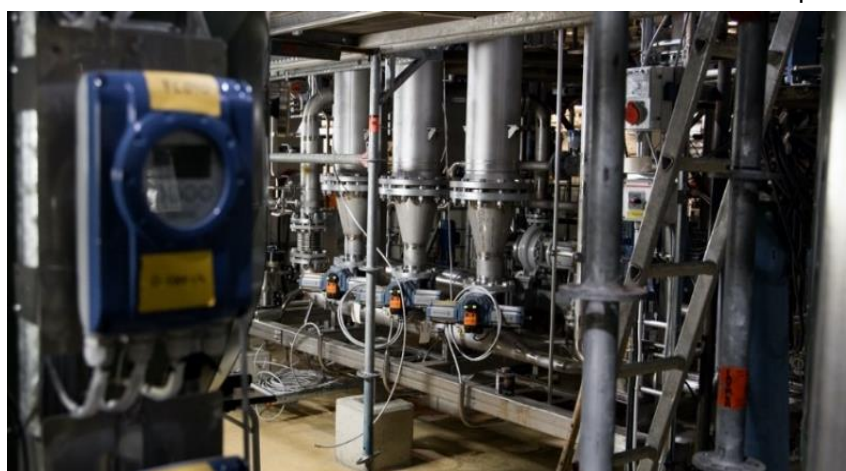
Figure 12 Ecohelix demo unit at the Domsjö mill in Sweden.
